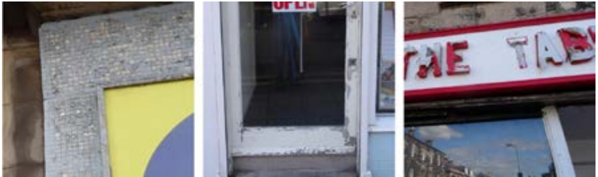
Lack of maintenance detracts from the overall attractiveness of the shopping area.
